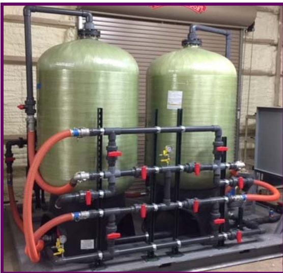
New system at IDA
